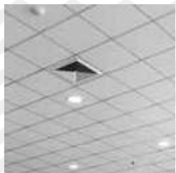
CEILING GRID FALSE CEILING
