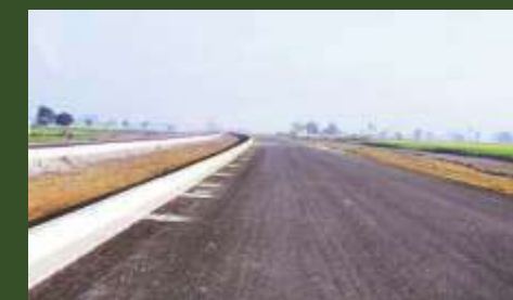
Actual photograph of the KMP expressway, nearing completion, close to the Raheja's Aranya City Site.
