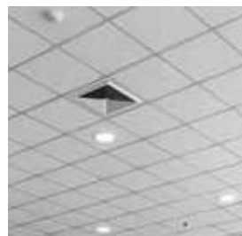
CEILING GRID FALSE CEILING
